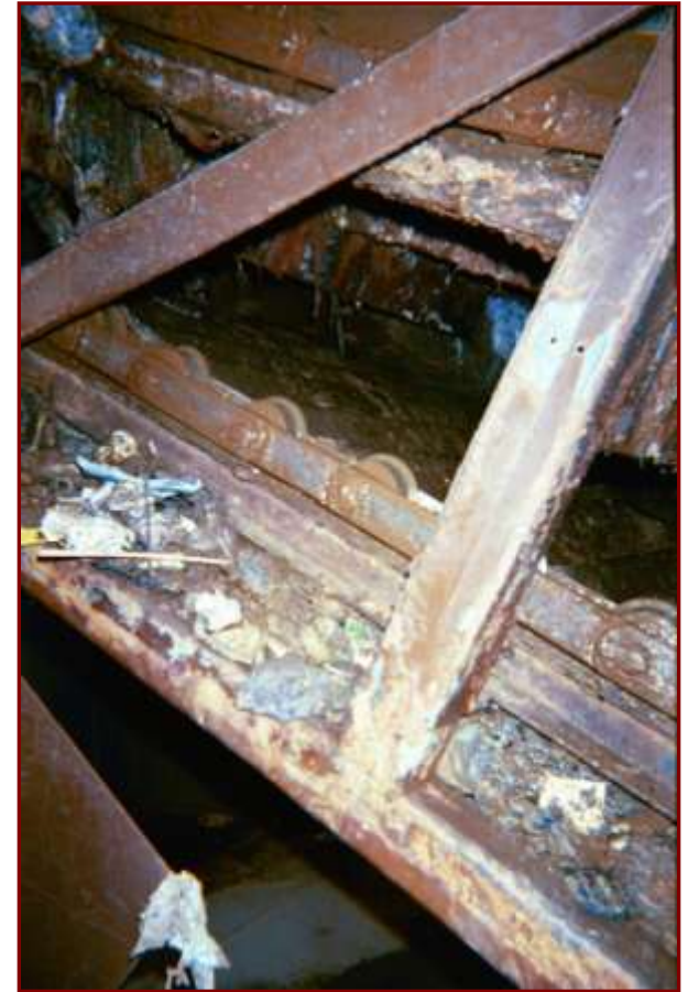
Premature Shaft Breakage
