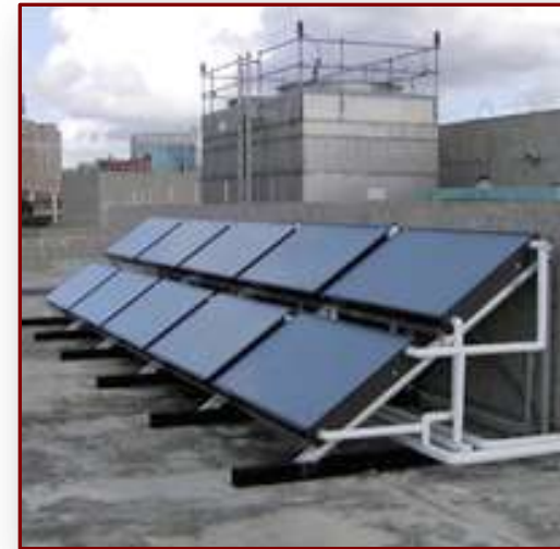
Solar Water Heating (reduce energy usage)
